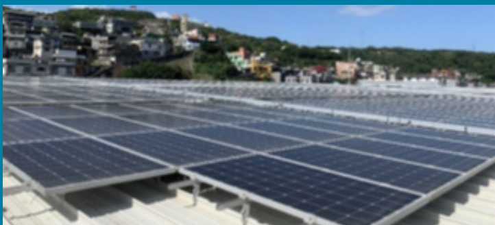
solar panels on the rooftop of West 7 warehouse
