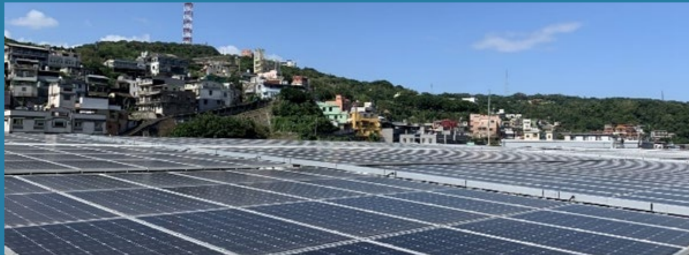
Solar panels on the roof of the West 7 warehouse
